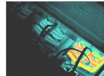
Above thermal image shows overheated windings on a step-down transformer, possibly caused by harmonics.
